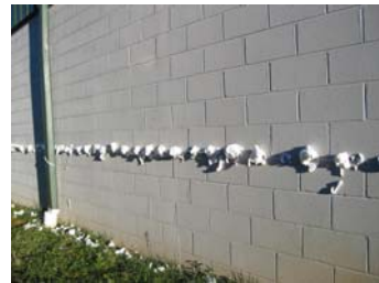
Drill-n-Fill or Pressure-Fill Where Foam is Injected via Small Holes in the Mortar Joints or CMU Face
